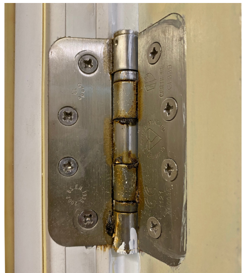
Hinges on potential fire or escape route doors which have become badly worn
