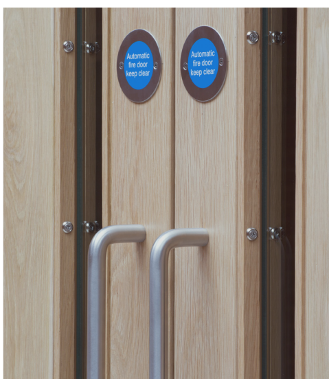
Pull handles on a fire door
